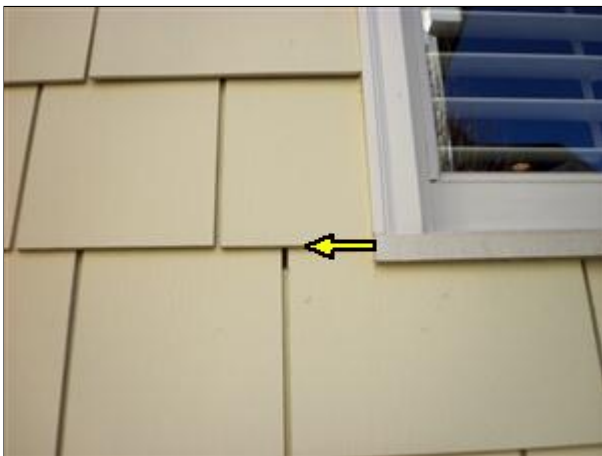
2.0 Picture 3 visible house wrap
