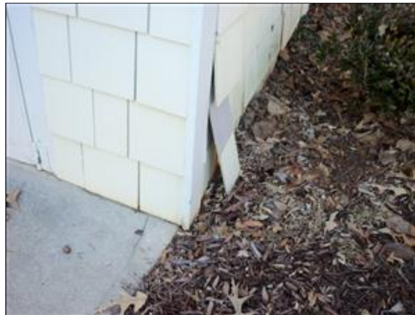
2.3 Picture 3 damage at corner - at ground level
