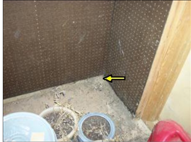
2.3 Picture 2 termite tubes
