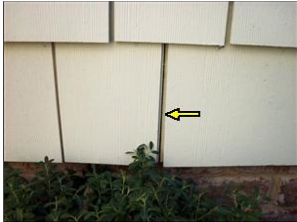
2.0 Picture 2 improperly aligned joints
